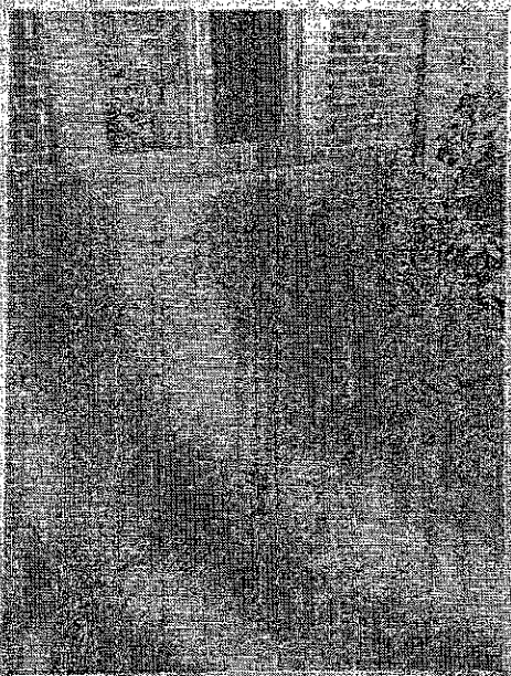
Front of house where leak occurred after repair
